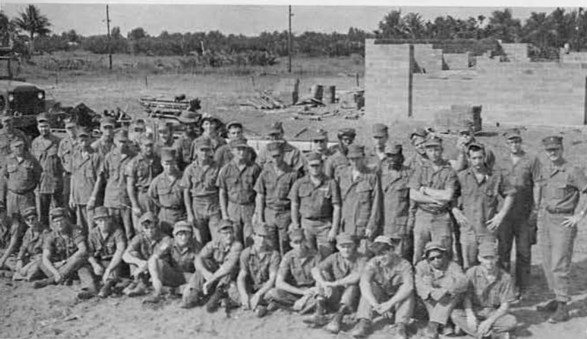
NAVCAT 14 at An Khan is engaged in Dependent Shelter Construction down the Delta region in support of the Vietnamese Navy.
